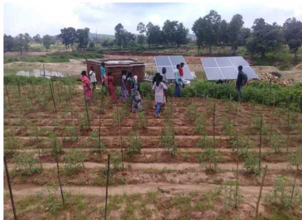
Solar Irrigation System at Churchu, Hazaribag
